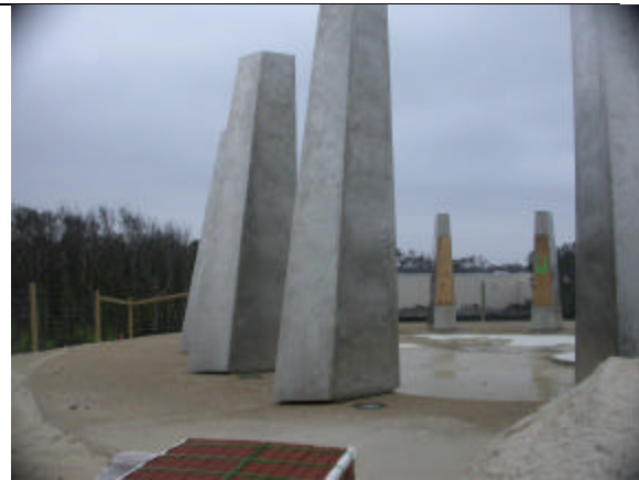
Coast Guard Pylon in Monument to A Century of Flight during construction at Kitty Hawk, N.C.
